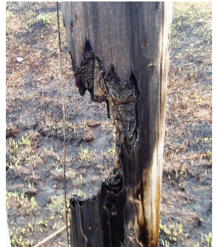
Before burning, check the property for electrical equipment and power poles to avoid damage and potential outages.
